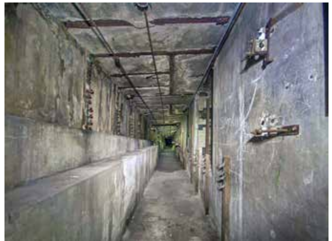
Power station cable duct
